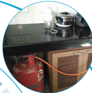
Gas Cylinders in Kitchen Area
